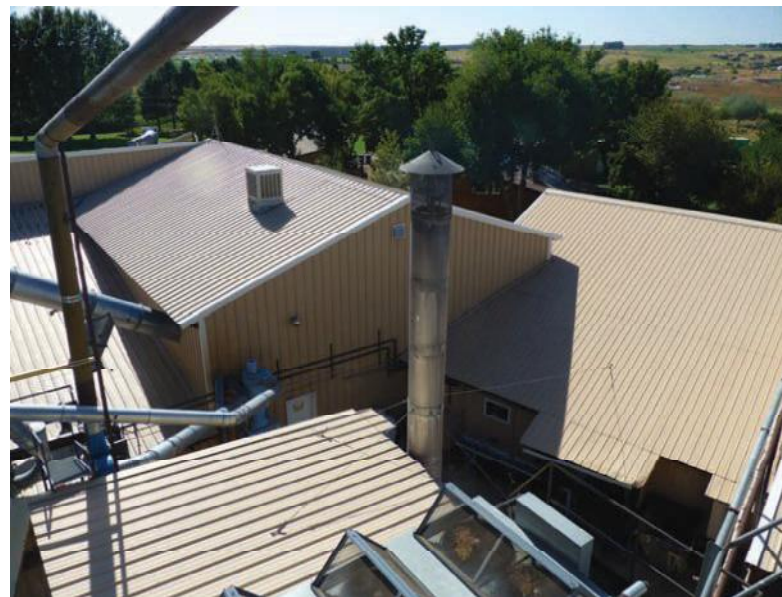
This view is from atop the silo at the Muscanell's facility near Cortez, CO.
